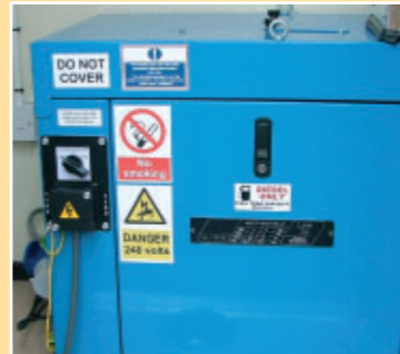
In-built PowACom diesel generator with voltage selector
