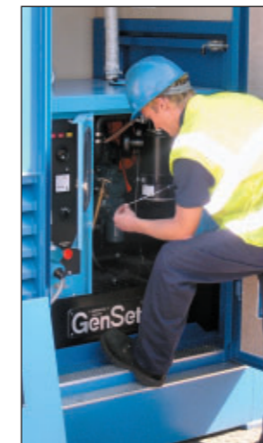
Easy access to generator for servicing and maintenance
