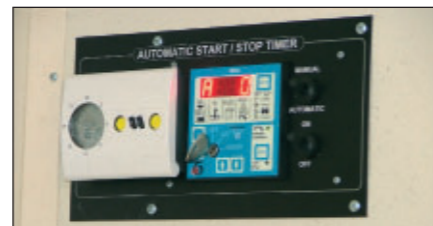
In-cabin automatic stop/start timer for generator
