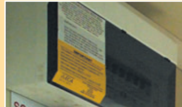
Electrical installation c/w certification
